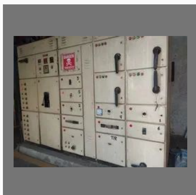
Electric Power Distribution Panel
