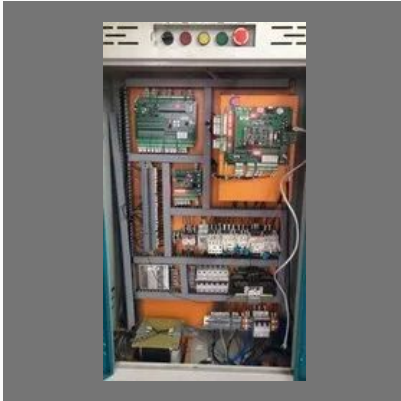
Automation PLC Control Panels
