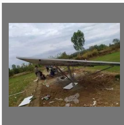
Solar Water Pumping System 3hp
