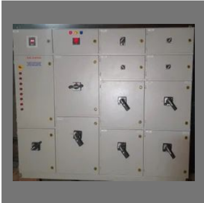
L.T Distribution With Apfc Panel
