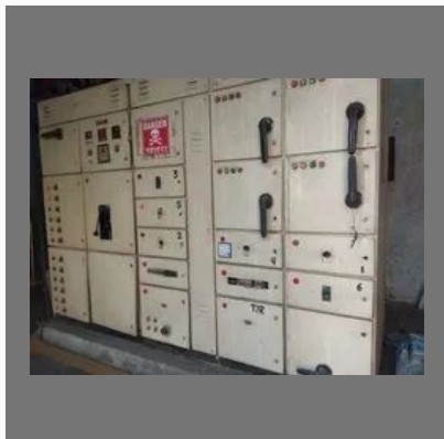
MCC Electrical Control Panel
