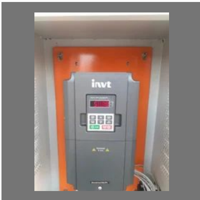
Solar Vfd Control Panel
