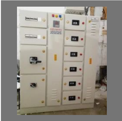
Power Distribution Board
