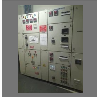
Automatic Control Panels
