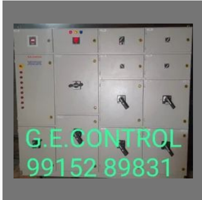
L.T Control Distribution Panel
