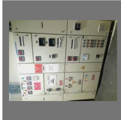
Power Control Center Panel
