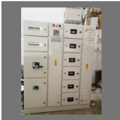
Power Control Panel Board
