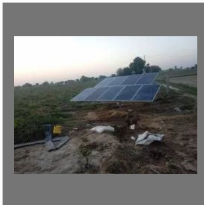
Solar Water Pumping System 7.5 Hp
