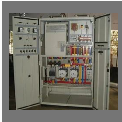
Automatic Changeover Panel
