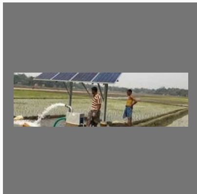
Shakti Solar Water Pump
