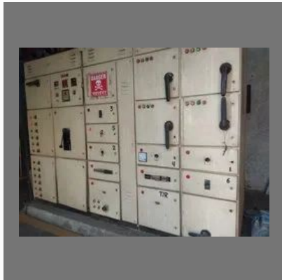
Electric Power Distribution Panel
