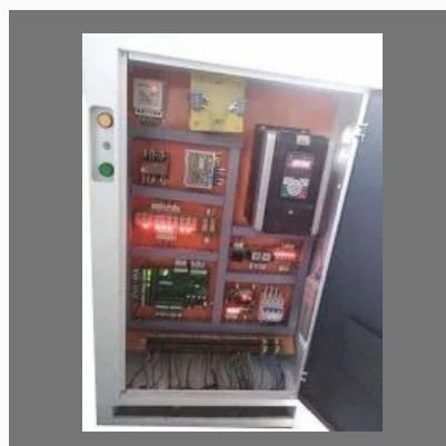
3HP Elevator Panels
